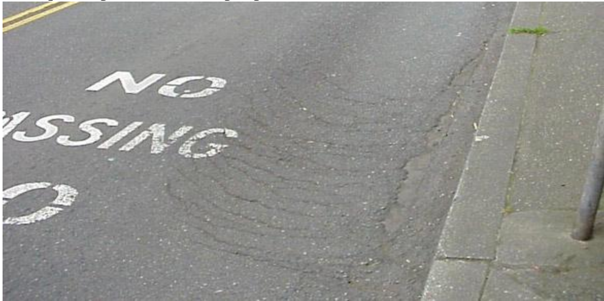
Fig. Slippage Cracks
