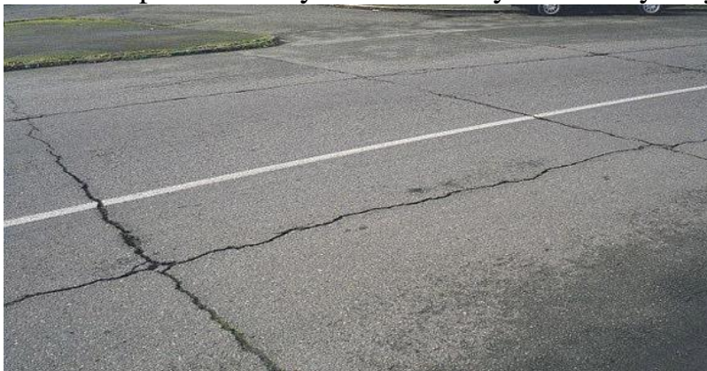
Fig. Joint Reflection Cracks
