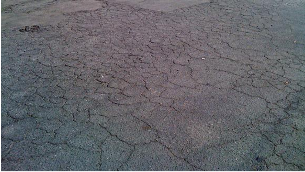
Fig. Alligator Cracking
