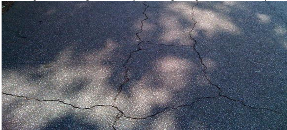
Fig. Block Cracking
