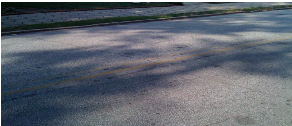
Fig. Transverse Cracking
